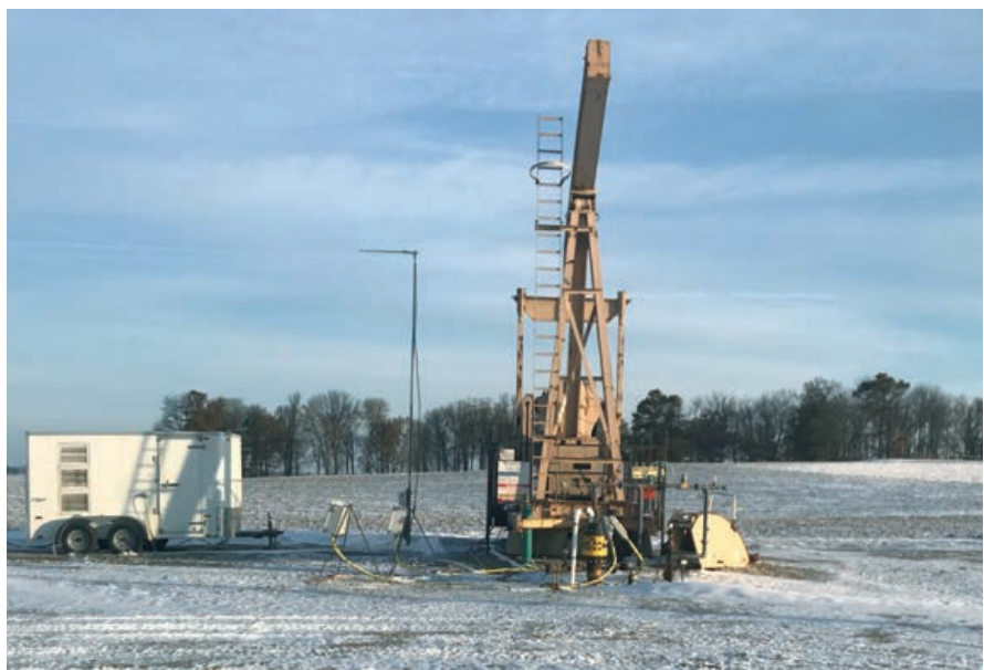
Top Side High Frequency Drive, Necessary Transformers, Communication and Safety Systems Located in Mobile Control Center Operate the SCS Motor without Sensors
